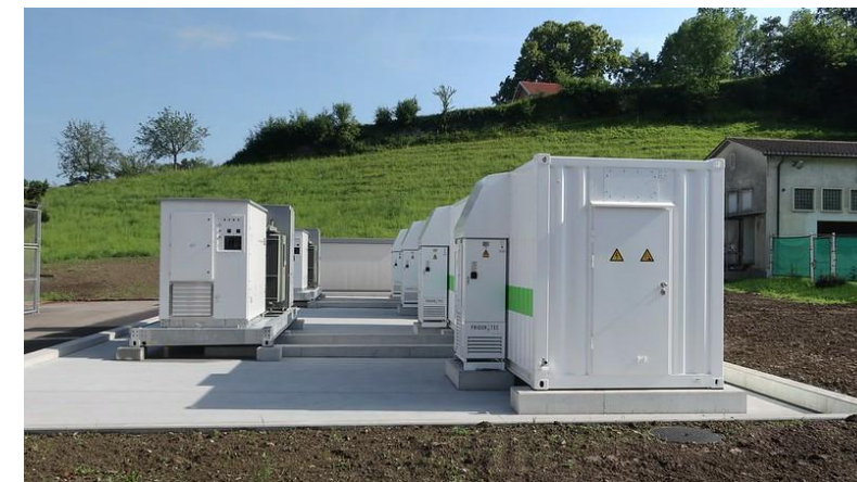
Image source : Rheineck Large Battery Storage Device https://www.flickr.com/photos/kecko/53777638626/in/photostream/
