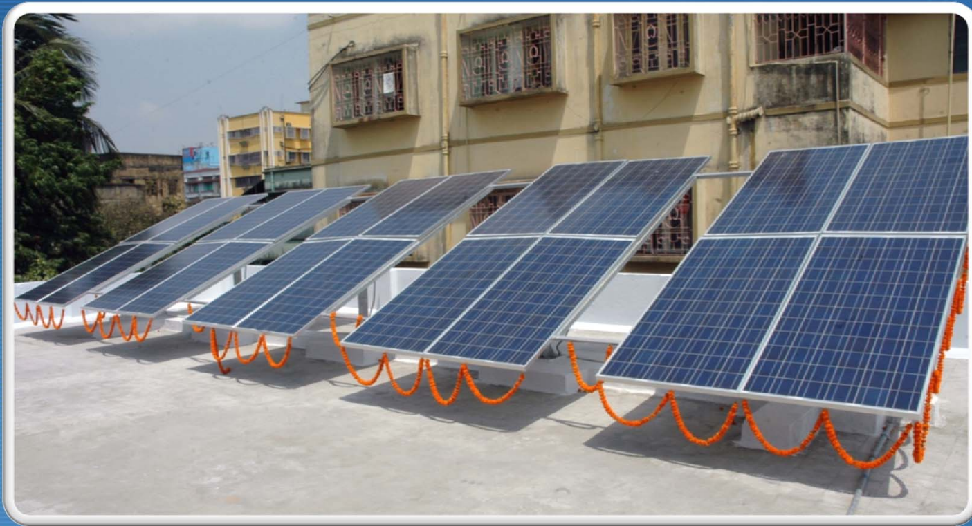
7.5 kw Grid Connected Roof Top Power Plant at Gurudas College, Kolkata
