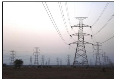
Transmission Lines Network in Chandrapur
