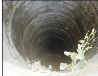
Dried well within 2 km from the coal mines
